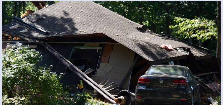
The Anne Arundel County Fire Department responded to an apparent explosion at a home in the Annapolis area. (Ulysses Muñoz/The Banner)
